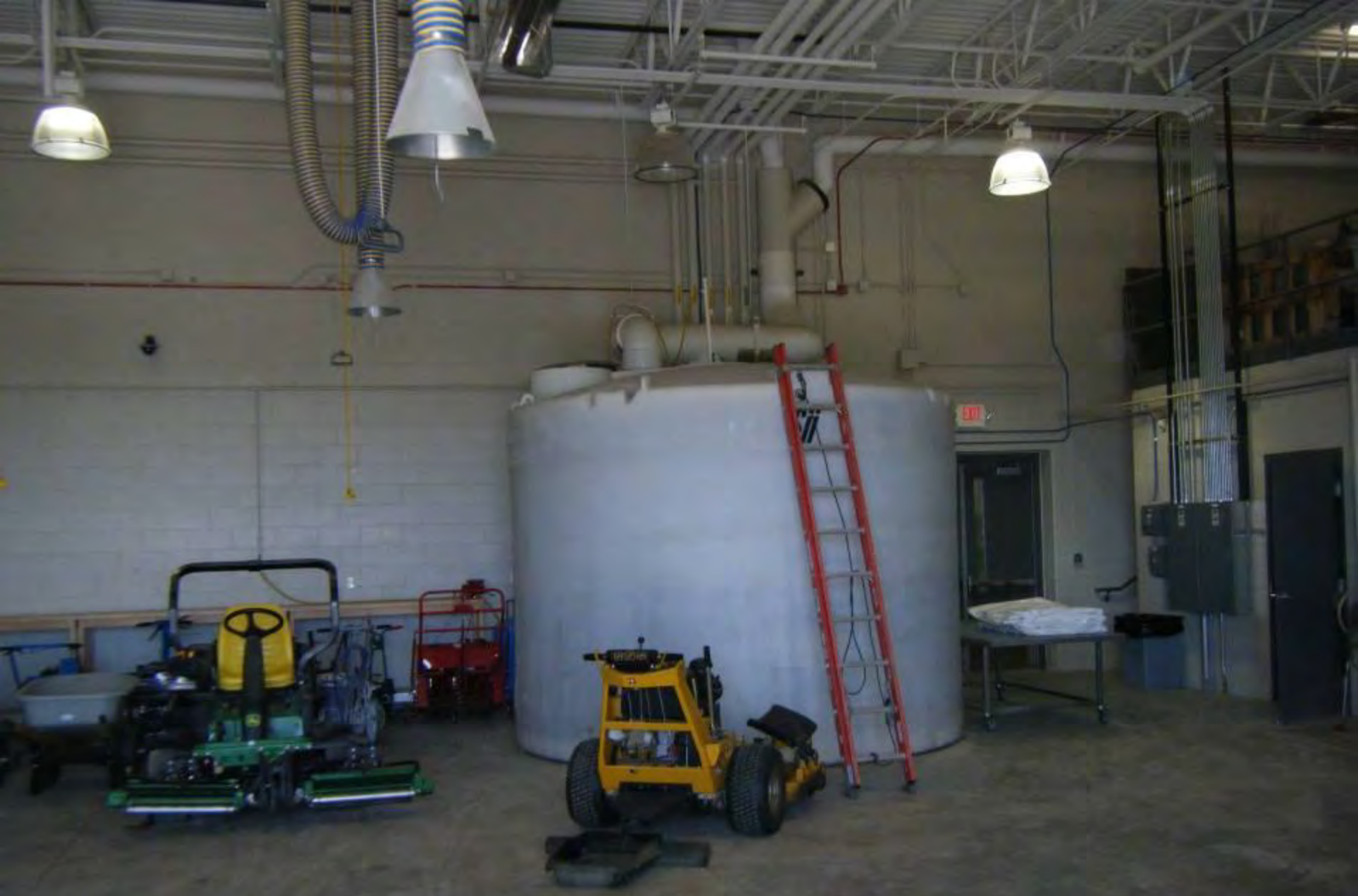
6,000 gal tank capturing roof water for greenhouse use at Kirkwood Community College in Cedar Rapids
