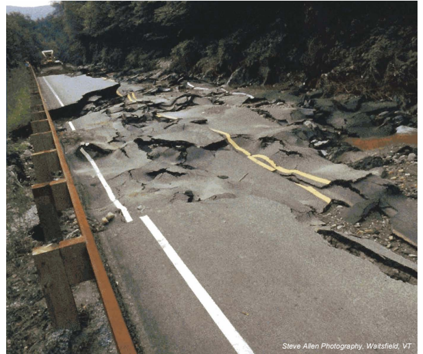
Road damage as a result of flash flooding.
