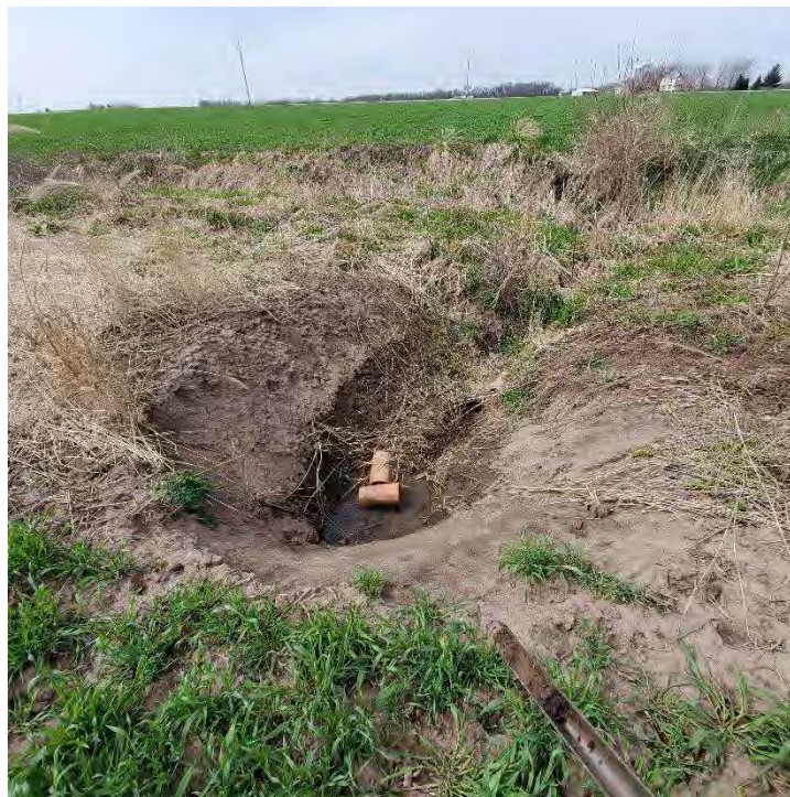
Photo 8: View looking northeast at apparent drainage tile discharging into Tributary 1 and Wetland 1.
