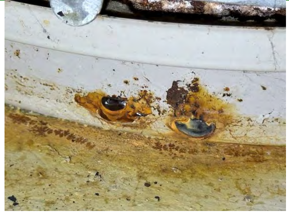
Unit # 6 Water Heater: RUST BUILD UP ON UNIT
