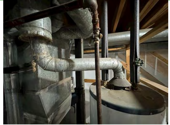
Unit # 14 Water Heater:
