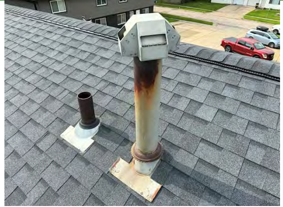
Unit # 6 Draft Control/Vent:
