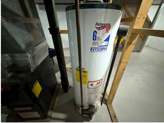
Unit # 14 Water Heater:
