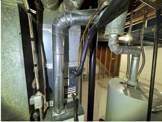
Unit # 1 Draft Control / Vent:
