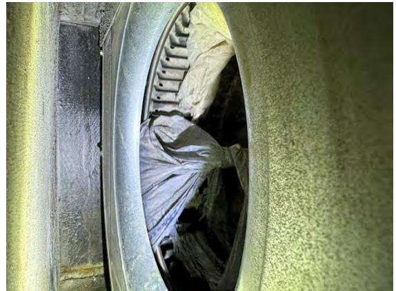
Unit # 3 HVAC Distribution: DEBRIS CAUGHT AND DIRTY BLOWER FINS
