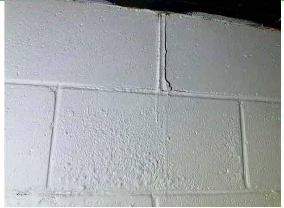
Unit # 1 Interior Foundation: GROUT LINE CRACKS AND PAINT BUBBLING
