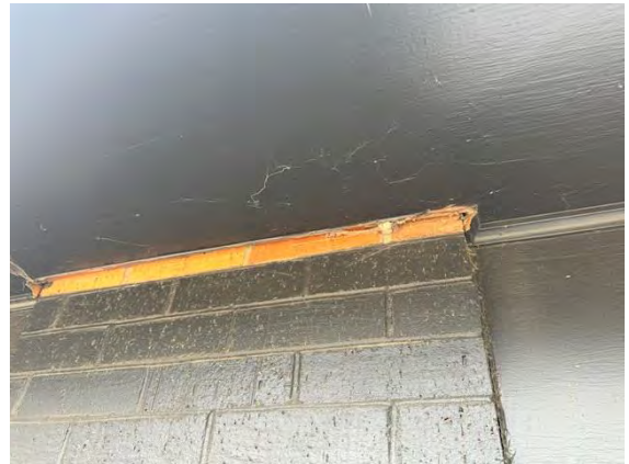
North Building Exterior Surface: MISSING WOOD TRIM
