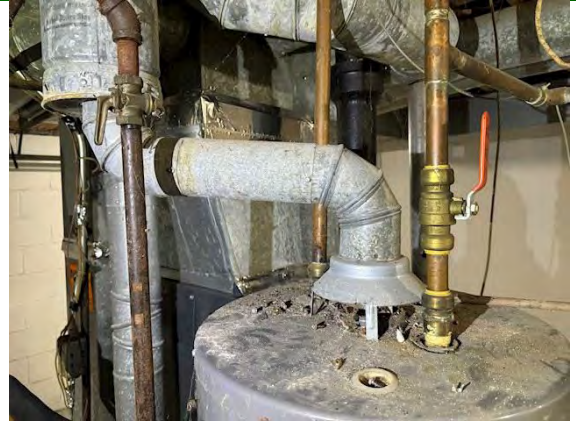
Unit # 10 Water Heater:
