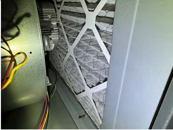
Unit # 11 HVAC Distribution:
