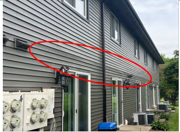
North Building Exterior Surface: BULGING SIDING
