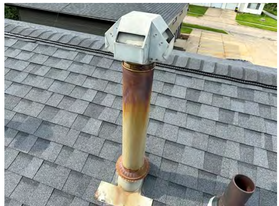
Unit # 10 Draft Control/Vent:
