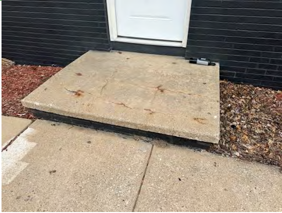
Complex Flatwork / Sidewalks: CRACKING AND GENERAL DETERIORATION OF ENTRYWAY SLAB
