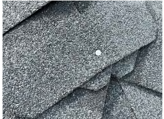
North Building Roofing: EXPOSED NAIL HEAD
