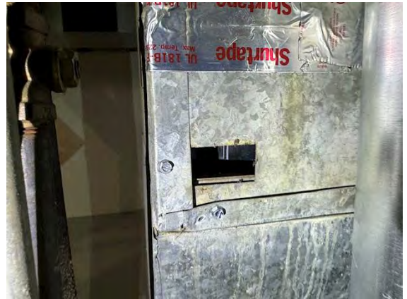
Unit # 5 HVAC Distribution: GAPS IN DUCT SYSTEM
