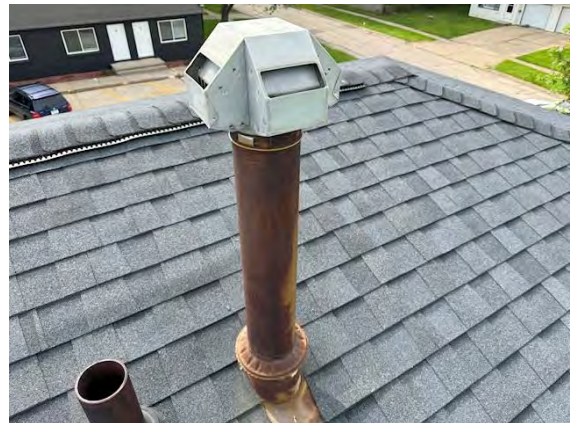
Unit # 2 Draft Control/Vent:
