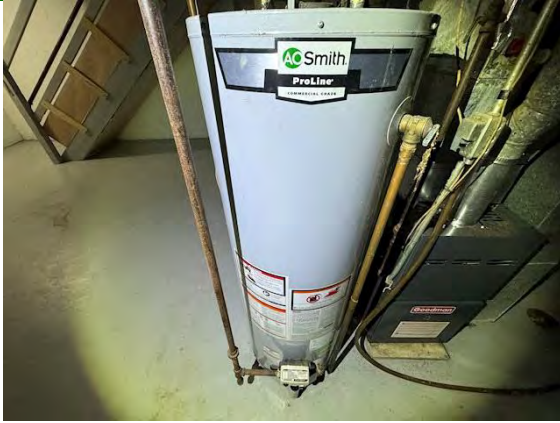
Unit # 7 Water Heater:
