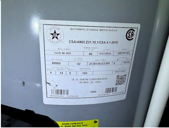
Unit # 3 Water Heater:
