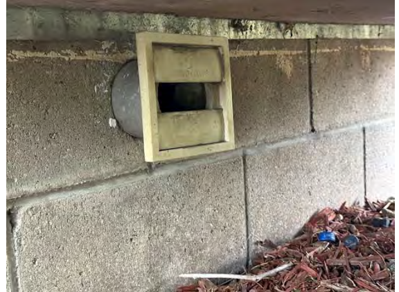
Laundry Facilities: DAMAGED DRYER VENT
