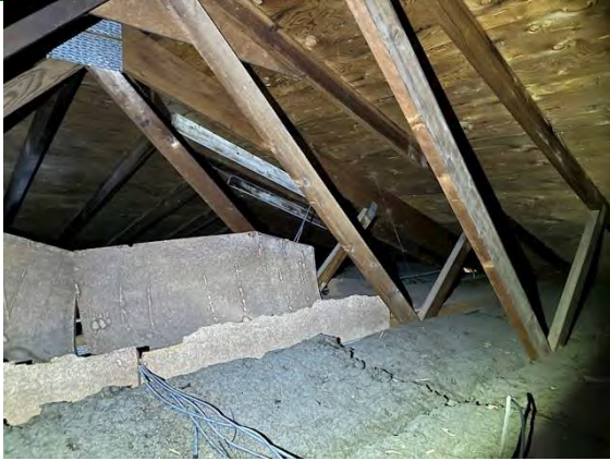
North Building Attic / Roof Framing and Sheathing: DAMAGED AND MISSING FIRE WALL
