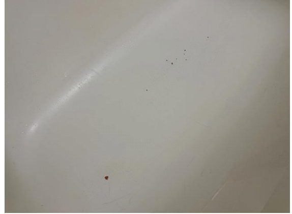
Unit # 2 Bathroom: CHIPPED AND DAMAGED ENCLOSURE
