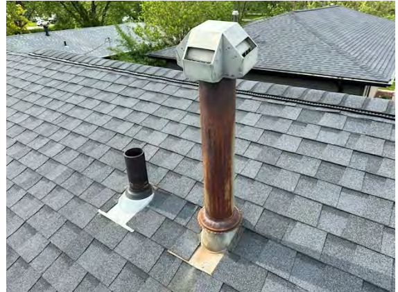
Unit # 9 Draft Control/Vent:
