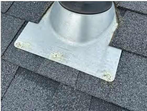
East Building Flashing / Valleys: CRACKED AND WEATHERED CAULKING
