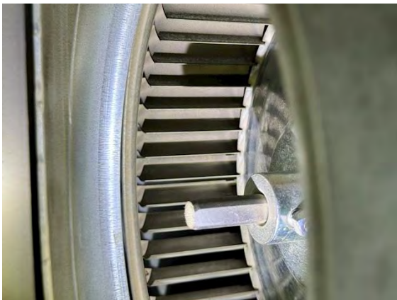
Unit # 2 HVAC Distribution:
