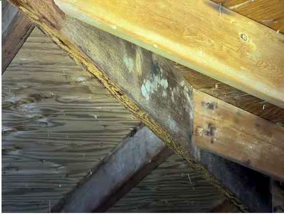
West Building Attic / Roof Framing and Sheathing: STAINING VISIBLE ON ATTIC FRAME WORK
