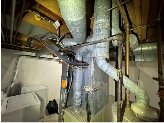
Unit # 6 Draft Control/Vent:
