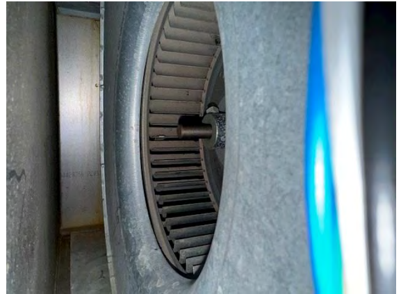
Unit # 13 HVAC Distribution:
