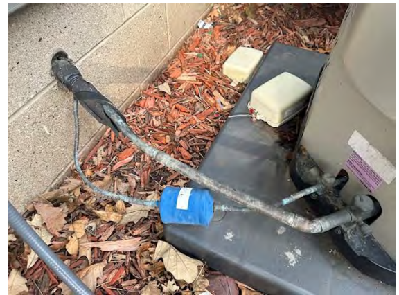
Unit # 5 Cooling: DAMAGED INSULATION
