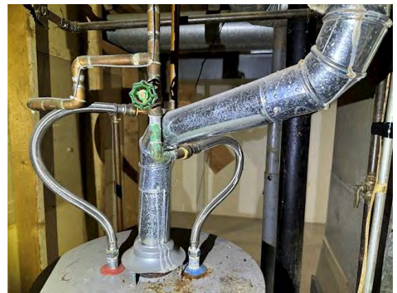
Unit # 5 Water Heater:
