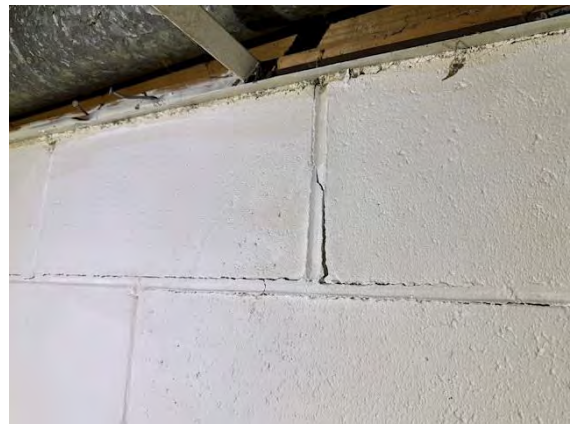
Unit # 2 Interior Foundation: GROUT CRACKS
