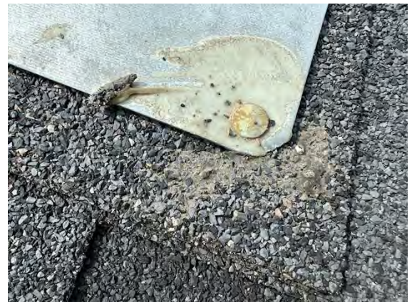
North Building Flashing/Valleys: EXPOSED NAIL HEAD
