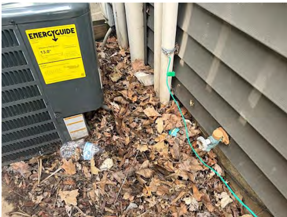
Unit # 12 Cooling: CLEAR LEAF DEBRIS FROM AWAY FROM UNIT
