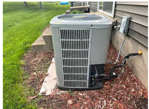
Unit # 4 Cooling: UN LEVEL SYSTEM
