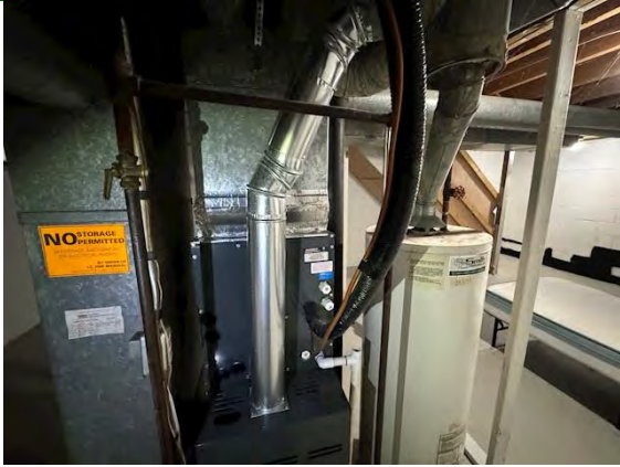
Unit # 12 Draft Control/Vent:
