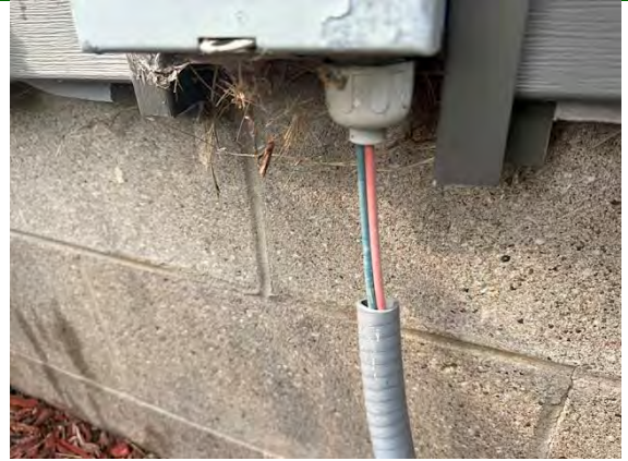
Unit # 4 Cooling: LOOSE CONDUIT AND EXPOSED WIRE
