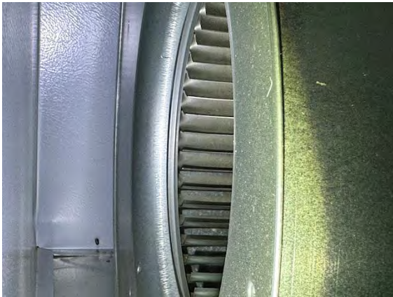
Unit # 5 HVAC Distribution:
