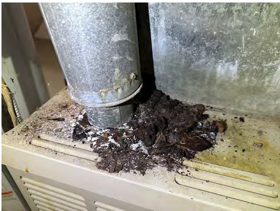
Unit # 15 Draft Control/Vent:
