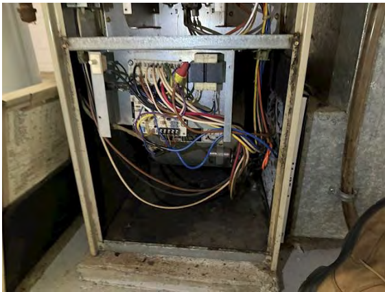
Unit # 15 HVAC Distribution:
