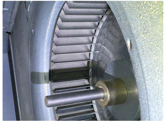
Unit # 1 HVAC Distribution:
