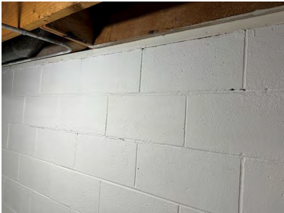
Unit # 5 Interior Foundation: GROUT CRACKS VISIBLE
