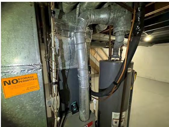
Unit # 10 Draft Control/Vent:
