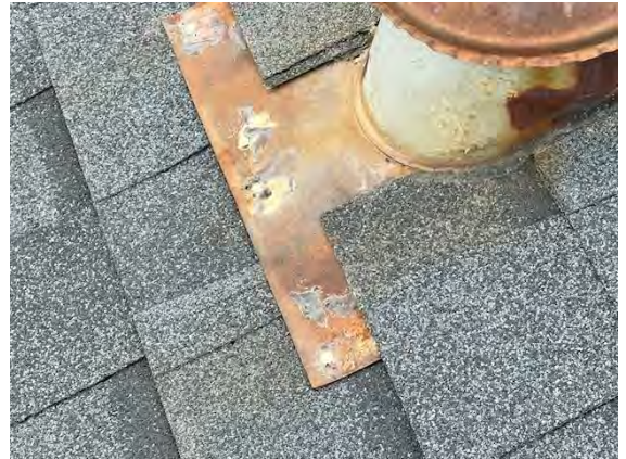
East Building Flashing / Valleys: RUSTED FLASHING
