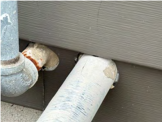
North Building Exterior Surface: UNCAULKED PENETRATIONS
