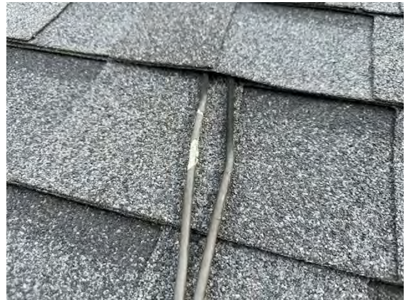
North Building Roofing: WIRES PENETRATING SHINGLES AND LAYING ON THE ROOF
