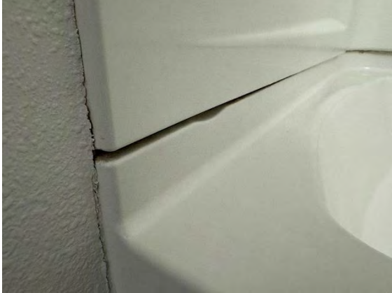
Unit # 1 Bathroom: GAPS IN SHOWER ENCLOSURE
