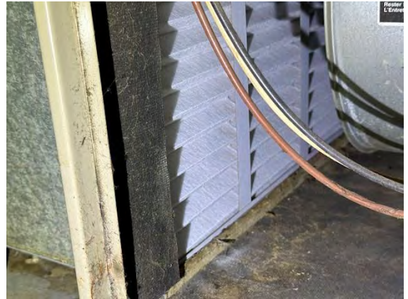
Unit # 8 HVAC Distribution:
