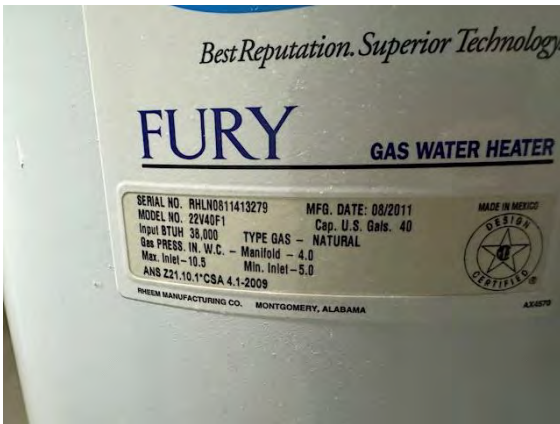
Unit # 15 Water Heater:
