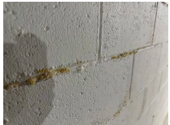
Unit # 15 Interior Foundation: EFFLORESCENCE
