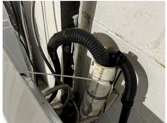
Sump/Sump Pumps Systems: UNIT 11 SUMP PUMP DISCHARGING INTO LAUNDRY
