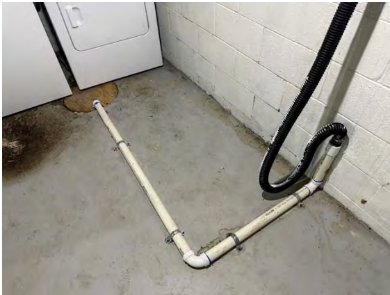
Sump/Sump Pumps Systems: SUMP PUMP DISCHARGE PIPE IN UNIT # 10
