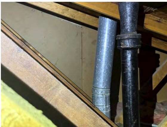
Unit # 8 Draft Control/Vent: LOOSE FLUE CONNECTIONS
