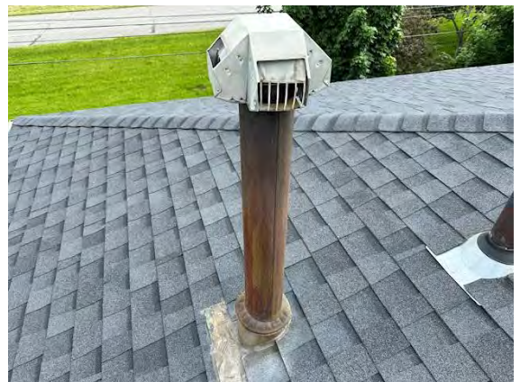
Unit # 4 Draft Control/Vent:
