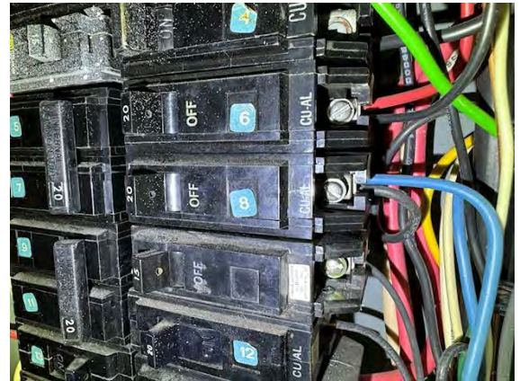
Unit #5 Electrical : DOUBLE TAPPED BREAKER
