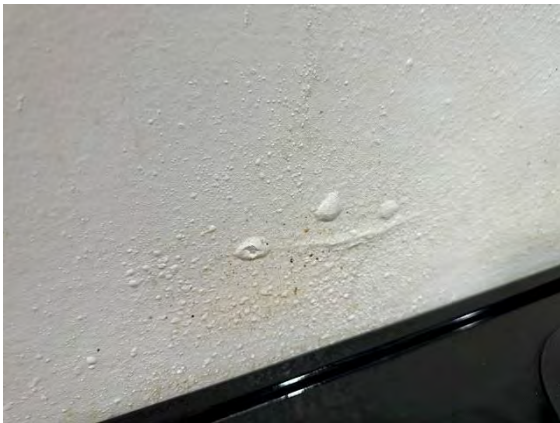
Unit # 5 Kitchen: WALL DAMAGE
