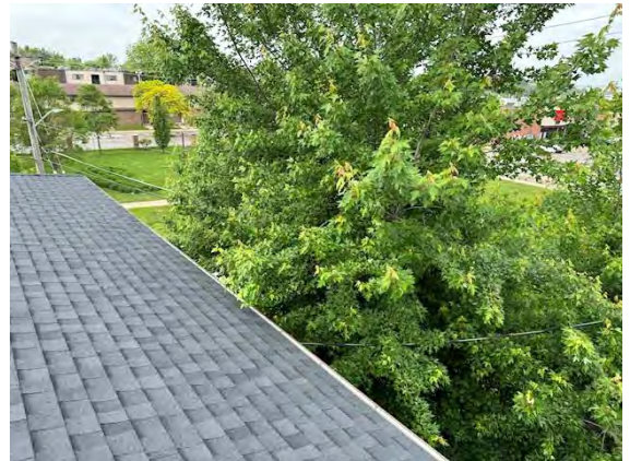
West Building Roofing: TREE IN CONTACT WITH ROOF
