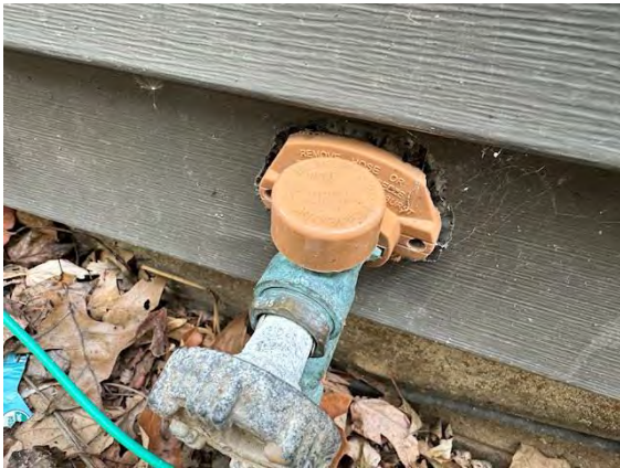
East Building Exterior Surface: UNCAULKED PENETRATIONS
