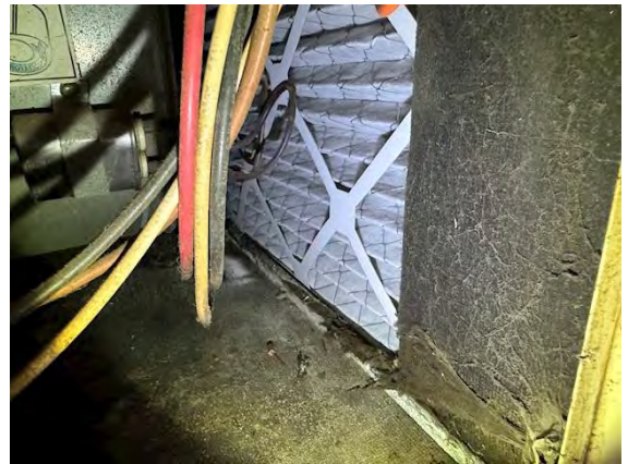
Unit # 15 HVAC Distribution:
