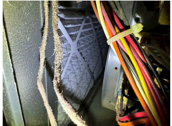
Unit # 14 HVAC Distribution:
