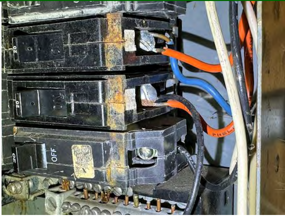
Unit #10 Electrical: DOUBLE TAPPED BREAKER
