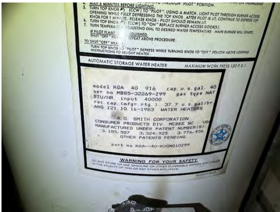
Unit # 12 Water Heater:
