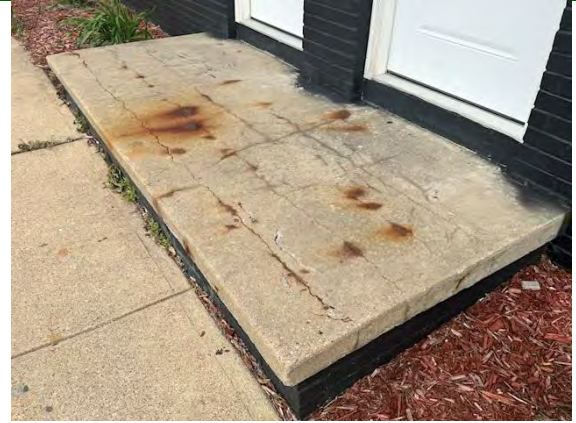
Complex Flatwork / Sidewalks: SETTLING AND DETERIORATION OF SLAB
