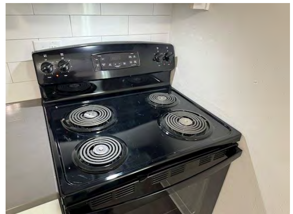
Unit # 1 Kitchen: STOVE IN DIRECT CONTACT WITH DRYWALL
