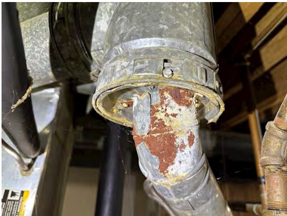
Unit # 8 Water Heater: RUST AND CORROSION
