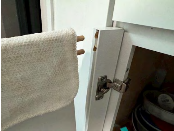
Unit # 9 Kitchen: DAMAGED / LOOSE CABINET DOOR
