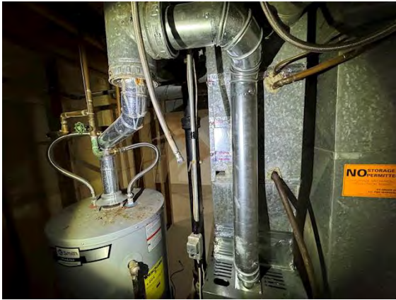
Unit # 5 Draft Control/Vent:
