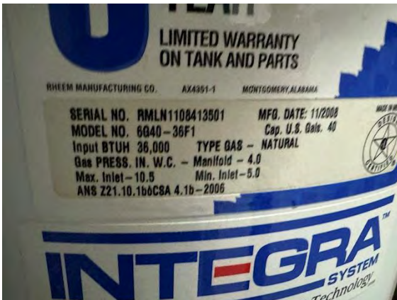
Unit # 14 Water Heater:
