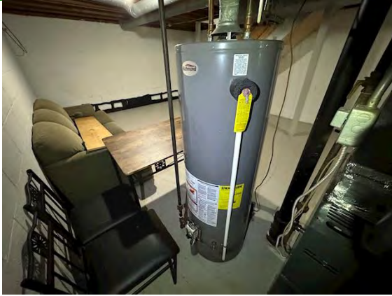
Unit # 11 Water Heater:
