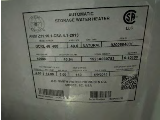
Unit # 1 Water Heater:
