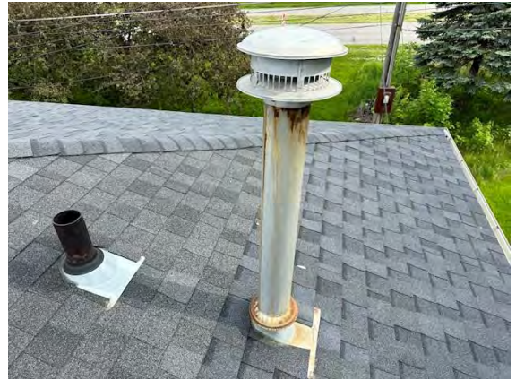
Unit # 11 Draft Control/Vent:
