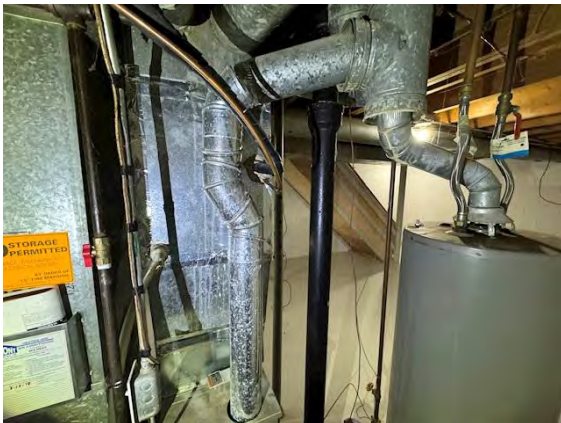
Unit # 2 Draft Control/Vent:
