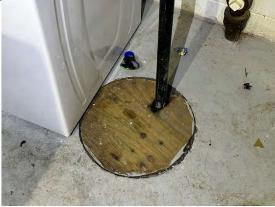
Sump/Sump Pumps Systems:
