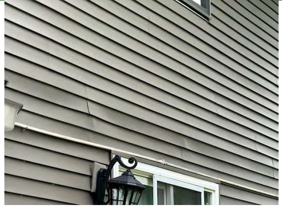
West Building Exterior Surface: LOOSE AND BULGING SIDING
