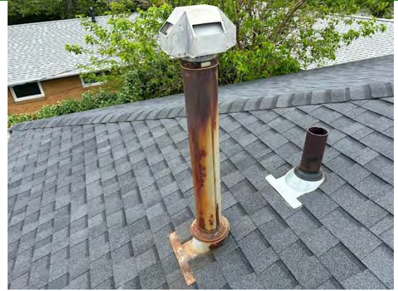
Unit # 12 Draft Control/Vent:
