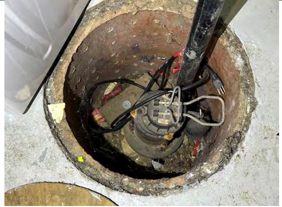
Sump/Sump Pumps Systems: UNIT #9
