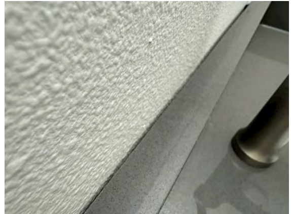
Unit # 1 Bathroom: CAULKING NEEDED ALONG BACKSPLASH
