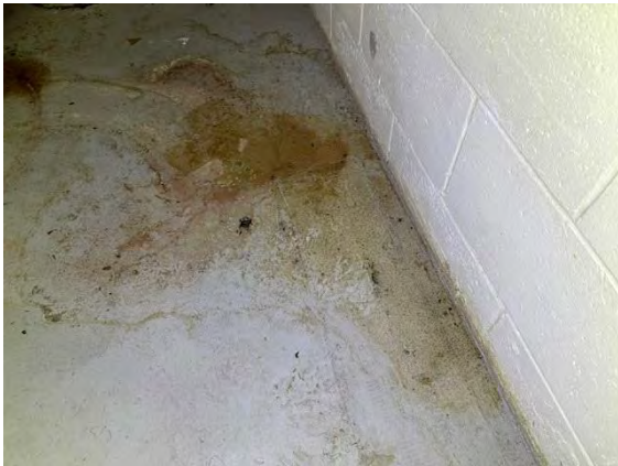
Unit # 9 Floor / Slab: ACTIVE WATER / MOISTURE
