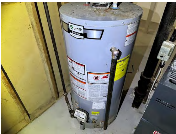
Unit # 5 Water Heater:
