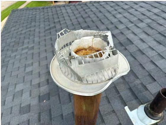
East Building Roofing: DAMAGED AND MISSING RAIN CAP
