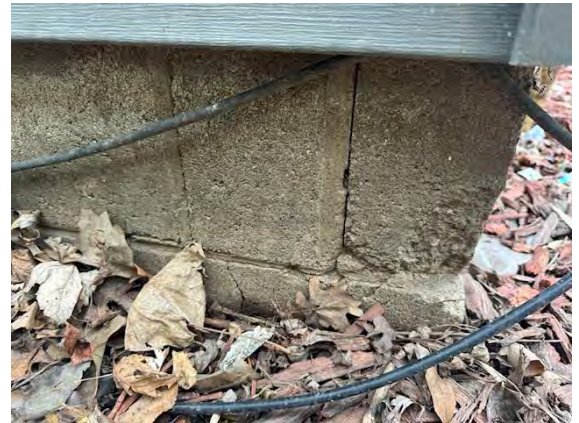
East Building Exterior Foundation: GROUT AND VERTICAL CRACKS IN FOUNDATION BLOCKS
