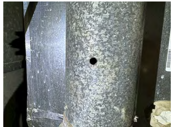
Unit # 8 Draft Control/Vent: TEST HOLE SHOULD BE SEALED
