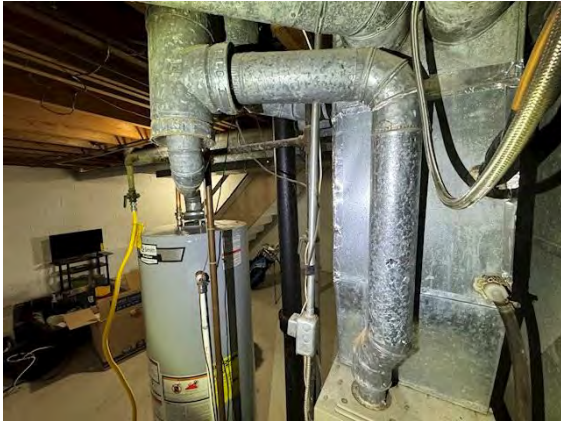
Unit # 3 Draft Control/Vent:
