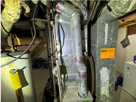
Unit # 9 Draft Control/Vent:
