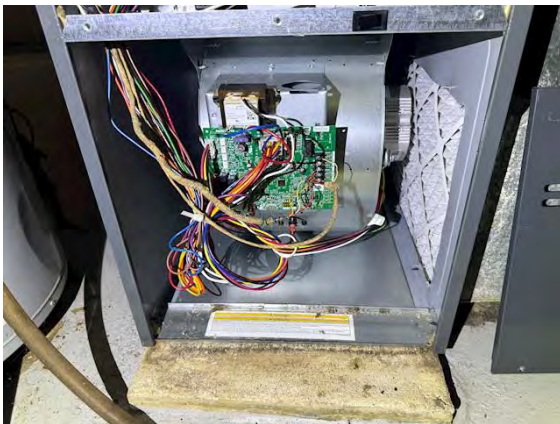
Unit # 7 HVAC Distribution:
