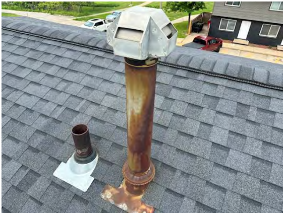
Unit # 14 Draft Control/Vent:
