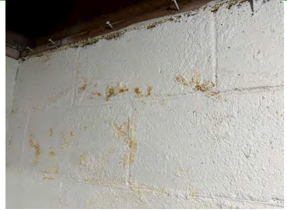
Unit # 14 Interior Foundation: EFFLORESCENCE
