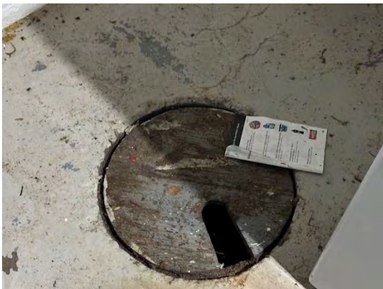
Sump/Sump Pumps Systems:
