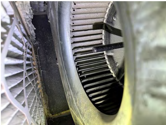
Unit # 6 HVAC Distribution: DIRTY BLOWER FINS
