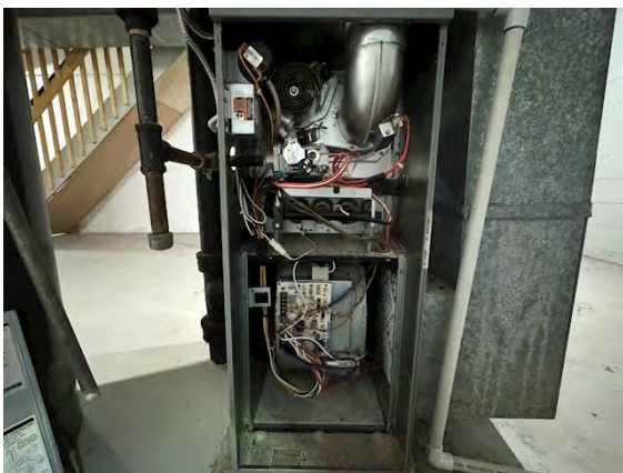
Unit # 13 HVAC Distribution:
