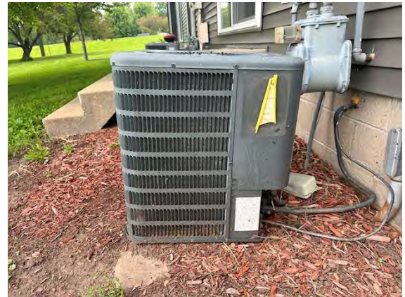
Unit # 1 Cooling: UN LEVEL AC UNIT
