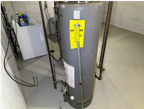
Unit # 2 Water Heater:
