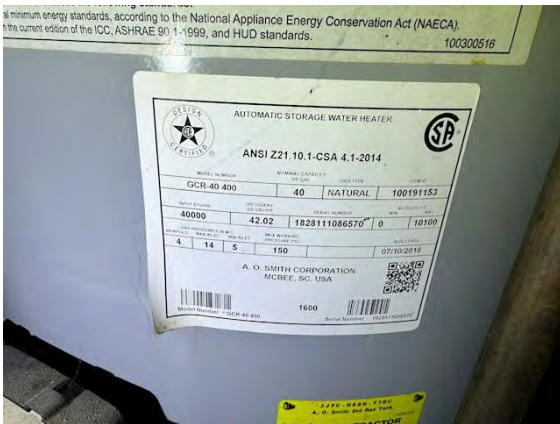
Unit # 7 Water Heater:
