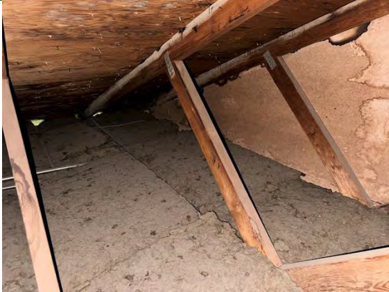
East Building Attic Ventilation: VENTILATION FROM THE SOFFITS WITH NO BAFFLES IN PLACE
