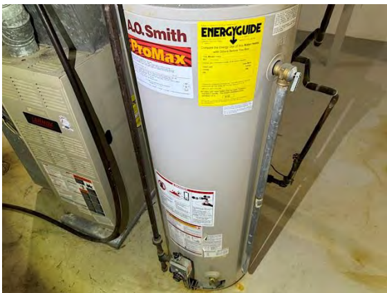
Unit # 6 Water Heater:
