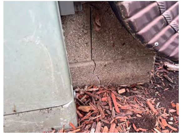
West Building Exterior Foundation: VERTICAL AND GROUT CRACKS IN FOUNDATION
