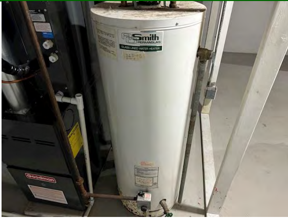
Unit # 12 Water Heater:
