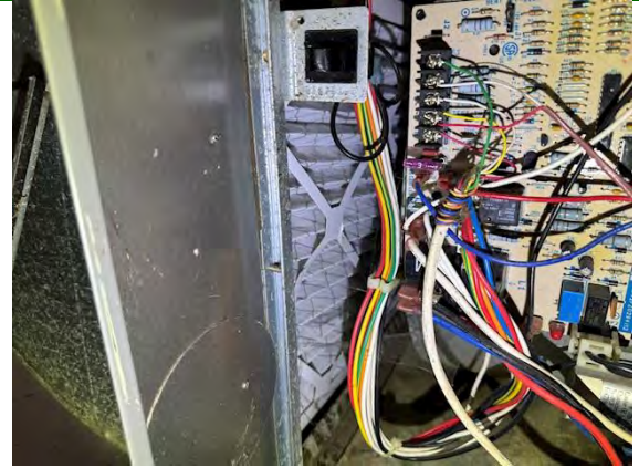
Unit # 10 HVAC Distribution:
