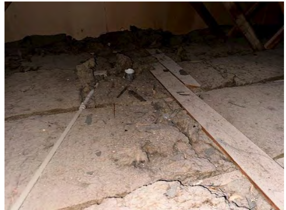
East Building Attic Insulation: STAINING ON INSULATION VISIBLE FROM BATHROOM VENTILATION
