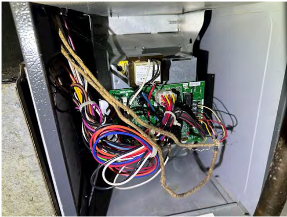
Unit # 1 HVAC Distribution:
