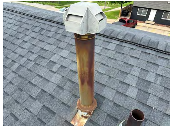
Unit # 13 Draft Control/Vent:
