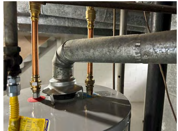
Unit # 3 Water Heater: NOT ENOUGH VERTICAL RISE
