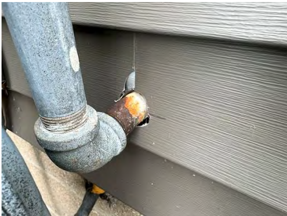
West Building Exterior Surface: UNCAULKED SIDING PENETRATIONS
