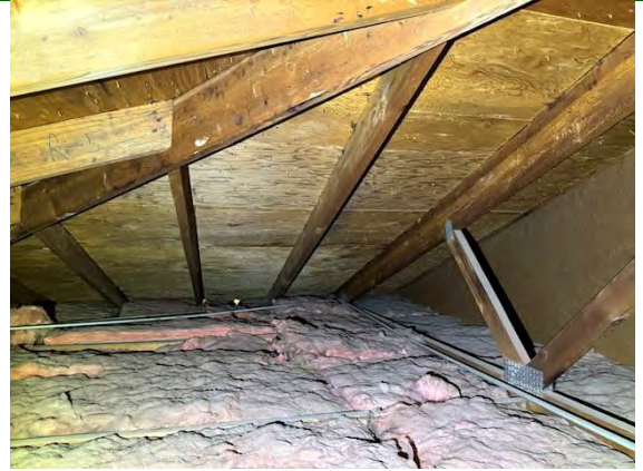
West Building Attic Ventilation: SOFFIT VENTS WITHOUT BAFFLES
