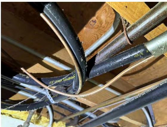
Unit # 9 Cooling: CONDENSATION FORMING ON SUCTION LINES
