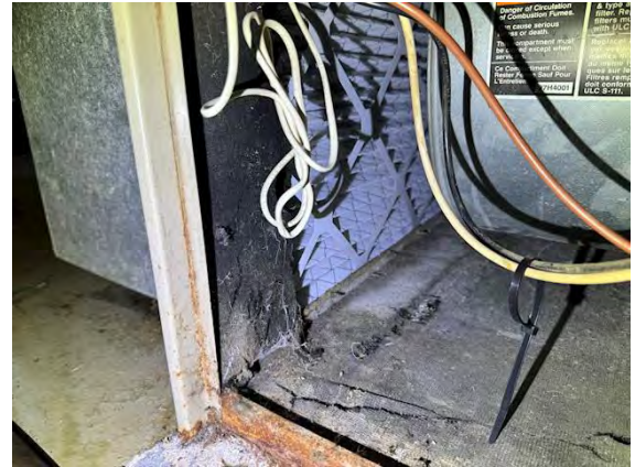
Unit # 6 HVAC Distribution:
