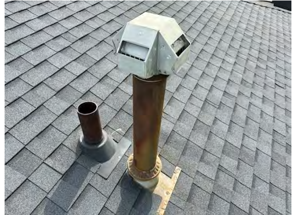
Unit # 3 Draft Control/Vent:
