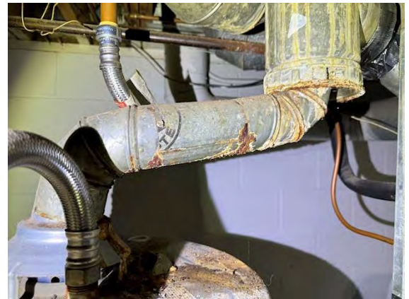
Unit # 4 Water Heater: NO 12" VERTICAL RISE
