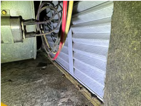
Unit # 3 HVAC Distribution:
