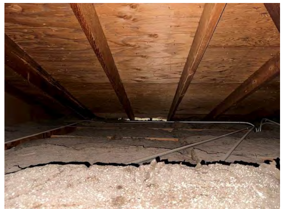
East Building Attic Ventilation: SOFFIT VENTILATION WITH NO BAFFLES INSTALLED
