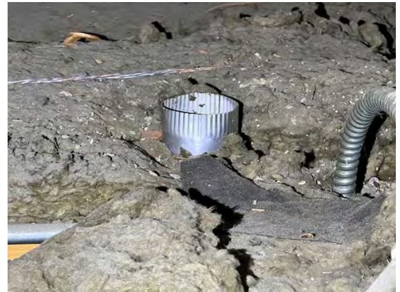
North Building Attic Insulation: MOISTURE STAINING AROUND BATHROOM VENT
