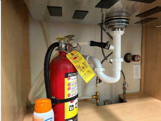
Unit # 12 Kitchen: NO DISHWASHER DRAINAGE LOOP
