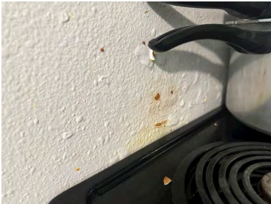
Unit # 9 Kitchen: DRYWALL DAMAGE DUE TO OVER PROXIMITY
