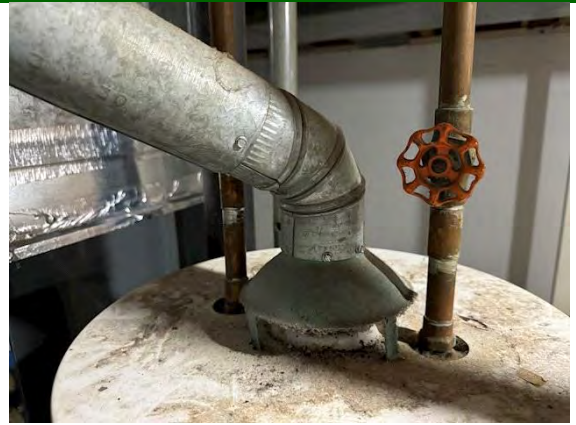
Unit # 12 Water Heater:
