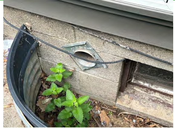
East Building Fenestration Systems: DRYER EXHAUST TERMINATING IN WINDOW WELL
