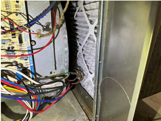
Unit # 13 HVAC Distribution:
