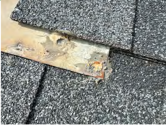
North Building Flashing/Valleys: RUSTED AND EXPOSED NAIL HEAD
