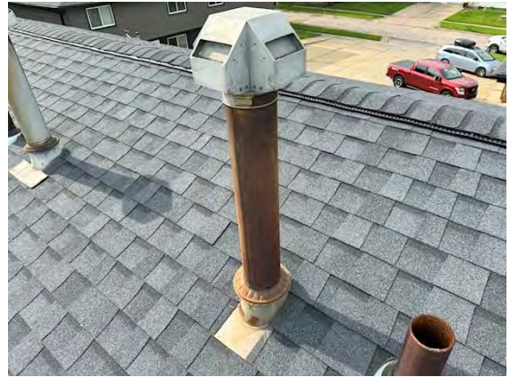
Unit # 5 Draft Control/Vent:
