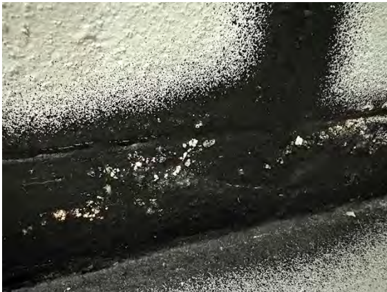
Unit # 12 Interior Foundation: EFFLORESCENCE
