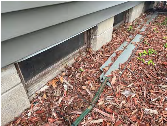
West Building Fenestration Systems: GRADE LEVEL WINDOWS WITH NO WINDOW WELLS
