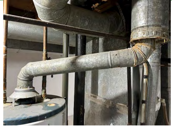
Unit # 15 Water Heater:
