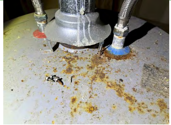
Unit # 5 Water Heater: RUST AND CORROSION ON TOP OF UNIT
