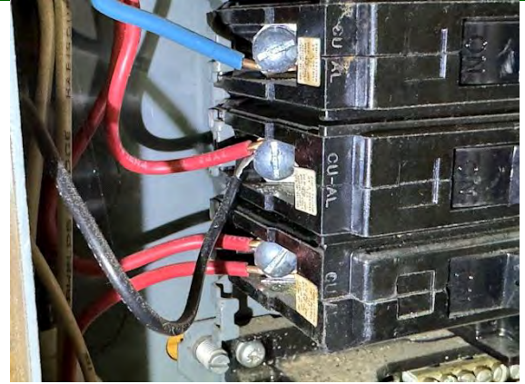
Unit #15 Electrical : DOUBLE TAPPED BREAKER
