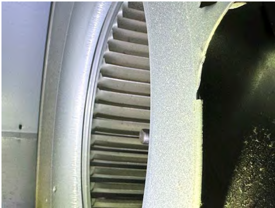
Unit # 4 HVAC Distribution:
