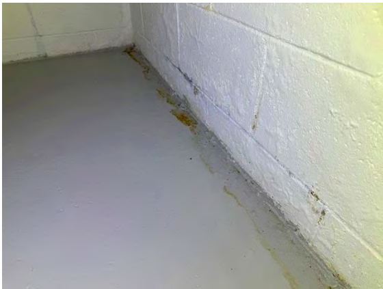
Unit # 1 Interior Foundation: SIGNS OF MOISTURE / ACTIVE WATER
