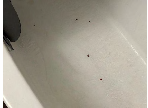
Unit # 9 Bathroom: CHIPS VISIBLE IN SHOWER ENCLOSURE
