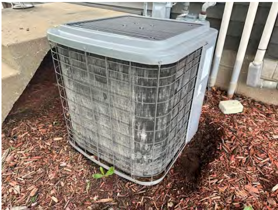
Unit # 2 Cooling: NO CONCRETE PAD INSTALLED
