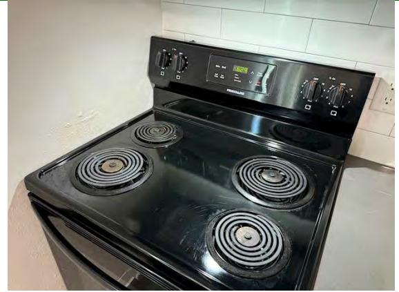
Unit # 5 Kitchen: STOVE INSTALLED NEXT TO DRYWALL
