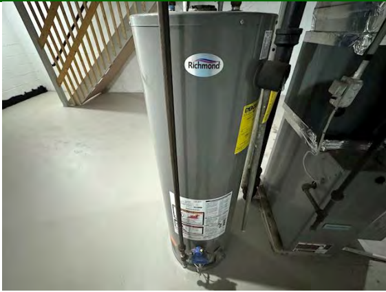
Unit # 13 Water Heater:
