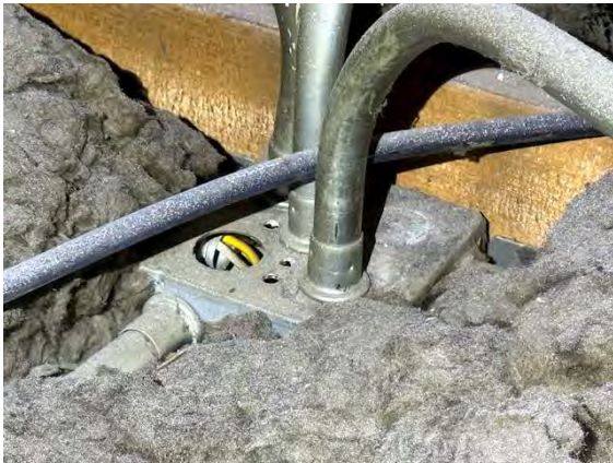
North Building Attic / Roof Framing and Sheathing: OPEN JUNCTION BOX
