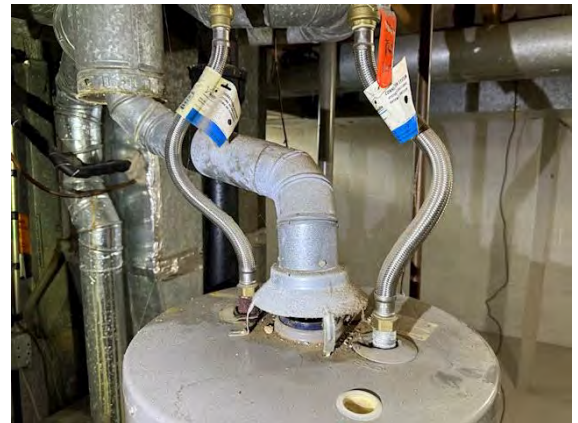
Unit # 2 Water Heater: LESS THAN 12" OF RISE
