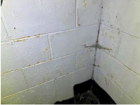
Unit # 1 Interior Foundation: EFFLORESCENCE
