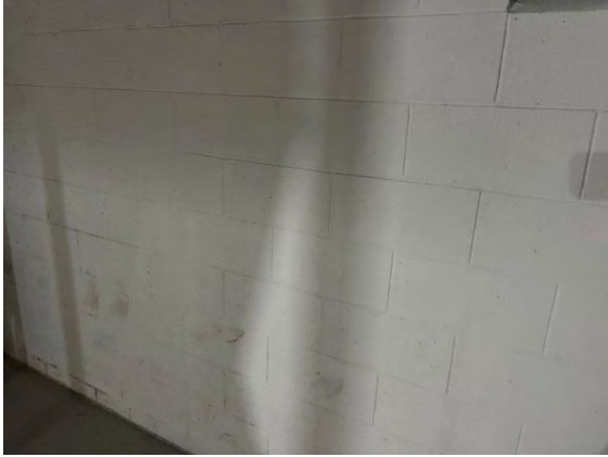
Unit # 12 Interior Foundation: EFFLORESCENCE
