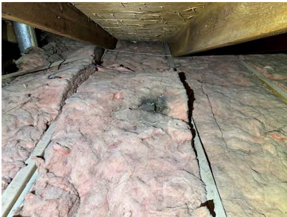
West Building Attic Ventilation: BATHROOM EXHAUST FAN VENTING INTO THE ATTIC WITH MOISTURE STAINING ON INSULATION
