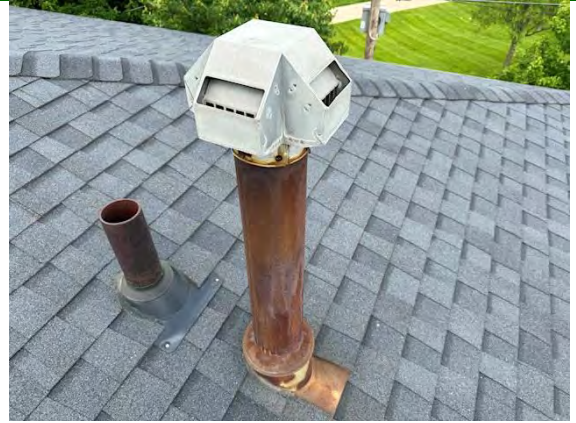
Unit # 1 Draft Control / Vent:
