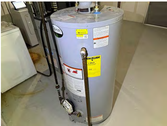
Unit # 1 Water Heater:
