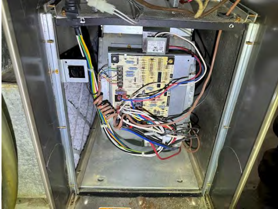
Unit # 2 HVAC Distribution:
