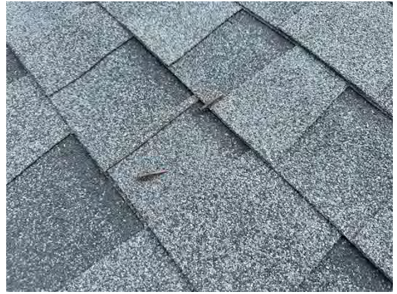
North Building Roofing: NAILS LEFT ON ROOF
