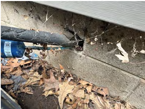
East Building Exterior Foundation: UNCAULKED PENETRATION
