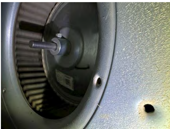
Unit # 14 HVAC Distribution:
