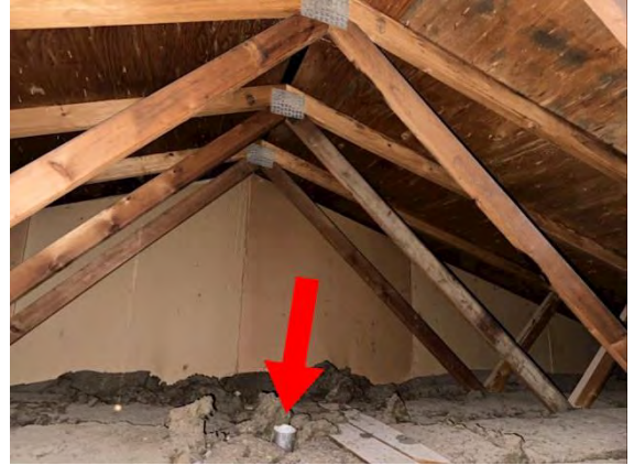
East Building Attic Ventilation: BATHROOM VENT TERMINATING IN ATTIC
