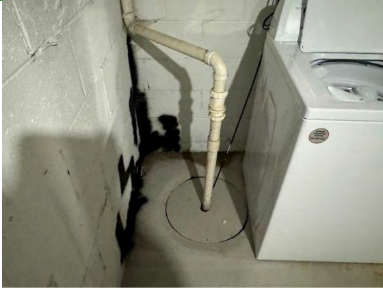
Sump/Sump Pumps Systems:
