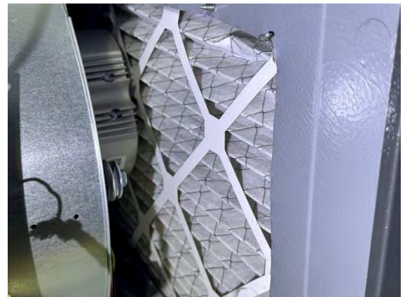
Unit # 7 HVAC Distribution:
