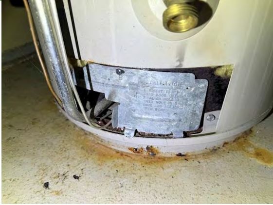
Unit # 6 Water Heater: MISSING COVER PLATE
