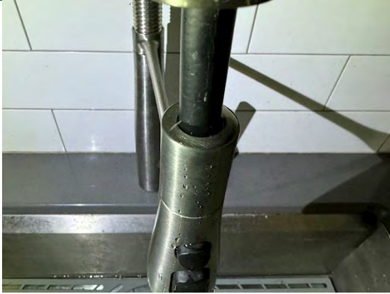
Unit # 2 Kitchen: FAUCET HEAD LEAKS
