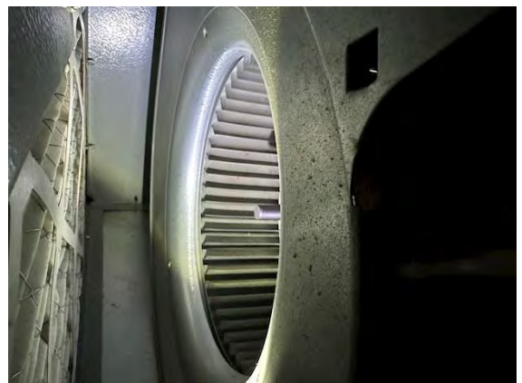
Unit # 12 HVAC Distribution:
