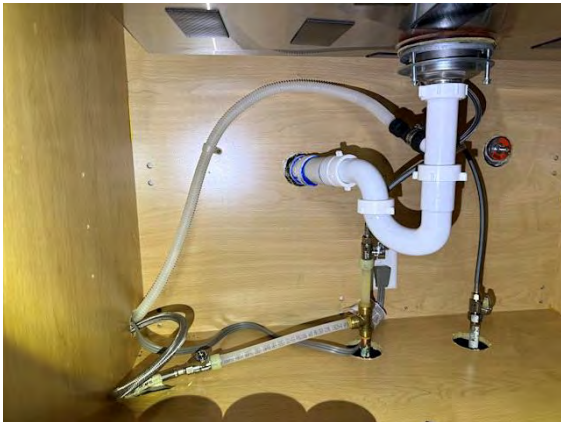
Unit # 2 Kitchen: DISHWASHER DRAINAGE LOOP NOT INSTALLED HIGH ENOUGH
