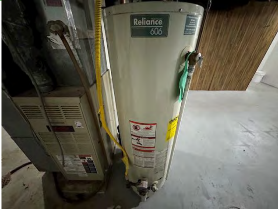
Unit # 8 Water Heater:
