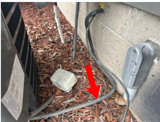
Unit # 1 Cooling: INSULATION MISSING FROM SUCTION LINE
