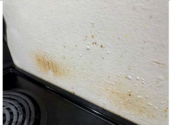
Unit # 4 Kitchen: BURN MARKS AND PAINT DAMAGE NEAR STOVE
