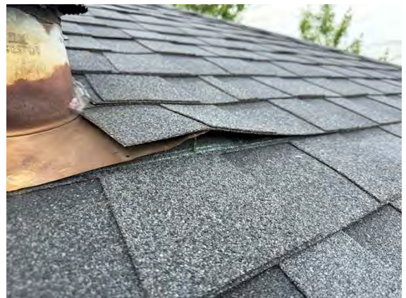
West Building Flashing/Valleys: RUSTED AND LIFTING FLASHING
