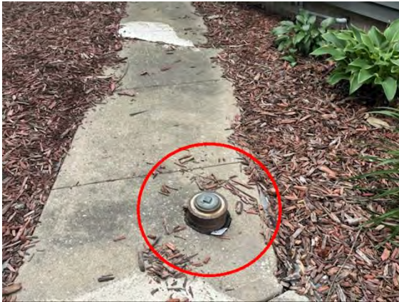
Complex Flatwork / Sidewalks: SETTLED WALKWAY WITH TRIPPING HAZARD
