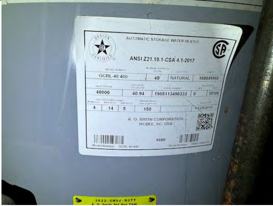
Unit # 5 Water Heater:
