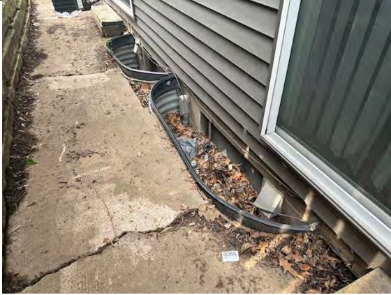
East Building Fenestration Systems: WINDOW WELL COVERS MISSING
