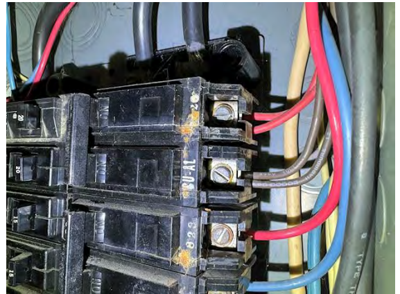
Unit #1 Electrical: DOUBLE TAPPED BREAKER
