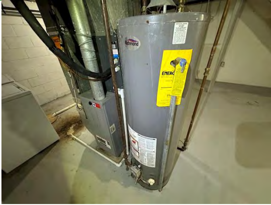
Unit # 10 Water Heater:
