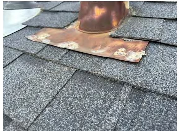
East Building Flashing / Valleys: RUSTED FLASHING
