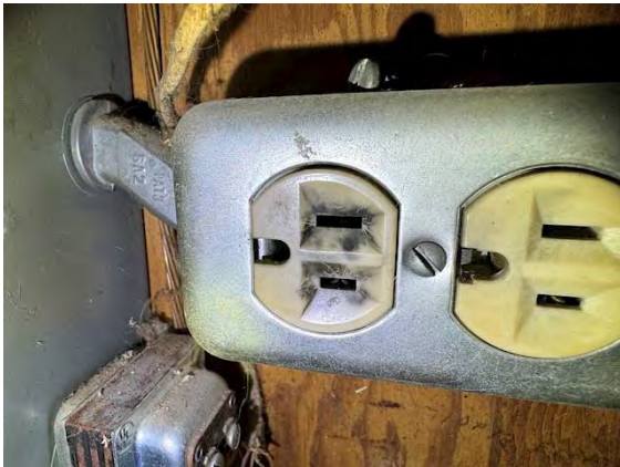
Unit #12 Electrical: SCORCHED AND DAMAGED OUTLET
