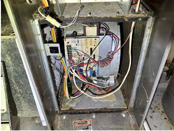
Unit # 10 HVAC Distribution:
