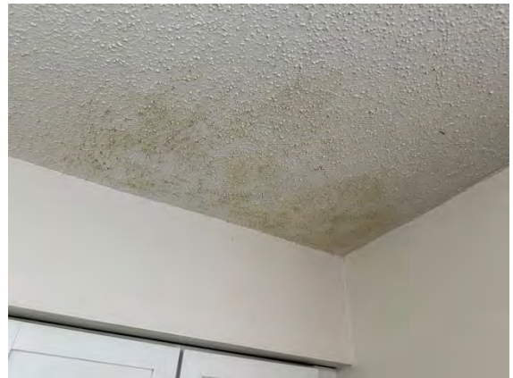
Unit # 4 Kitchen: CEILING STAINS
