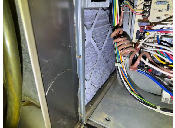
Unit # 2 HVAC Distribution:
