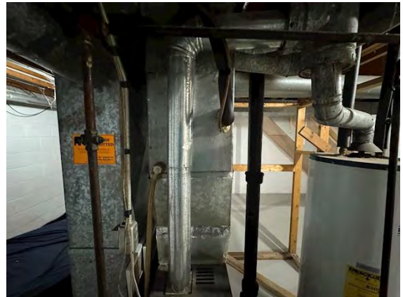
Unit # 14 Draft Control/Vent:
