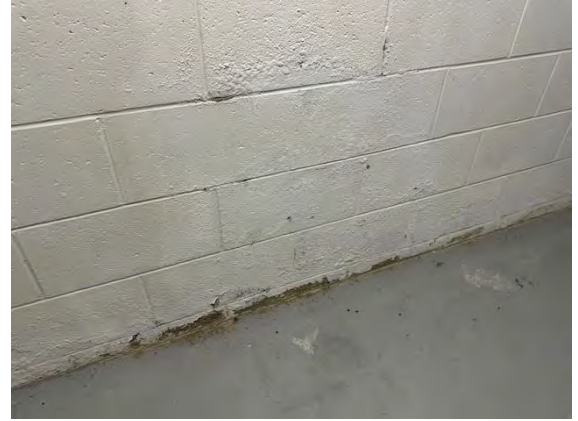
Unit # 8 Interior Foundation: SIGNS OF PREVIOUS MOISTURE AND EFFLORESCENCE
