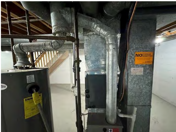
Unit # 13 Draft Control/Vent:
