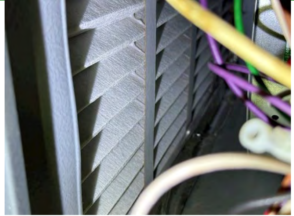
Unit # 4 HVAC Distribution:
