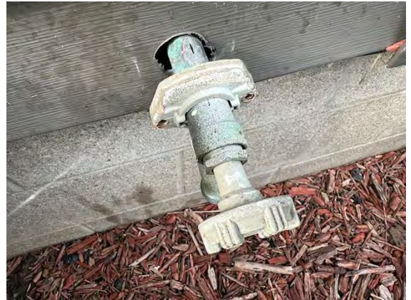
North Building Exterior Surface: LOOSE AND BURST EXTERIOR FAUCET
