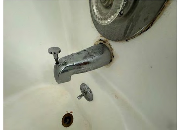
Unit # 4 Bathroom: LOOSE FAUCET HEAD
