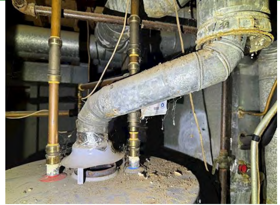
Unit # 7 Water Heater: VERTICAL RISE UNDER 12"
