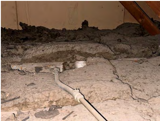
East Building Attic Insulation: STAINING ON INSULATION
