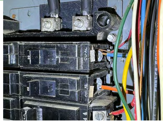
Unit #4 Electrical: LOW VOLTAGE WIRE DOUBLE TAP
