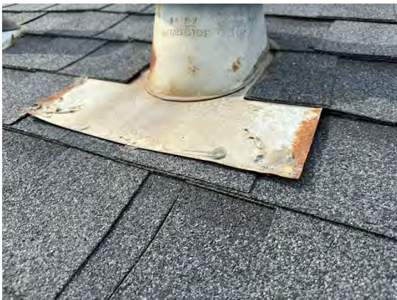
North Building Flashing/Valleys: RUSTED AND LIFTING FLASHING
