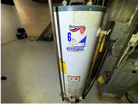
Unit # 9 Water Heater:
