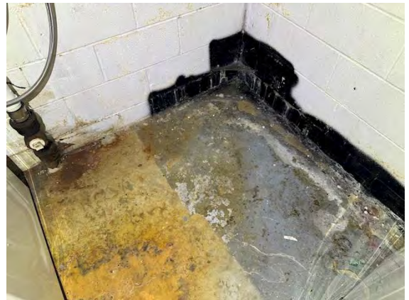
Unit # 1 Interior Foundation: MOISTURE AND PAST REPAIRS
