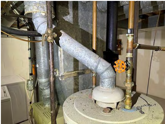
Unit # 6 Water Heater: NO VERTICAL RISE
