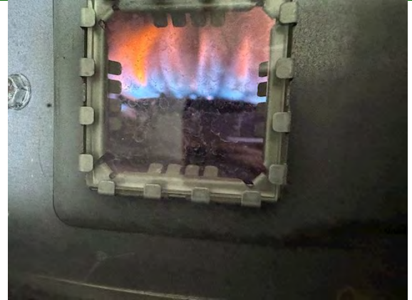
Unit # 1 Water Heater:
