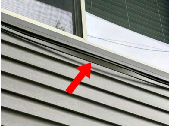
West Building Exterior Surface: LOOSE SIDING TRIM
