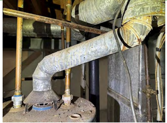
Unit # 9 Water Heater:
