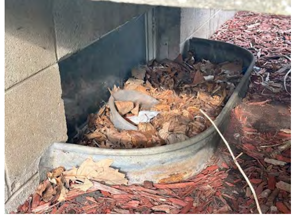
North Building Fenestration Systems: NO WINDOW WELL COVER AND FILLED WITH DEBRIS
