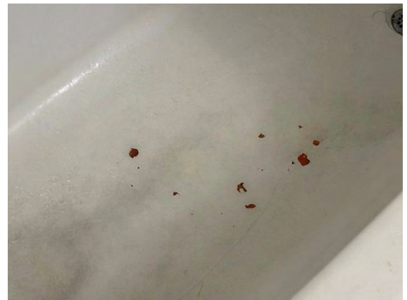
Unit # 10 Bathroom: DAMAGED ENCLOSURE
