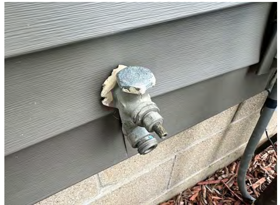
West Building Exterior Surface: MISSING HANDLE ON EXTERIOR FAUCET
