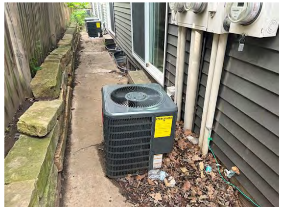
East Building Grading / Drainage: DEBRIS AND BUILD UP ALONG GRADE
