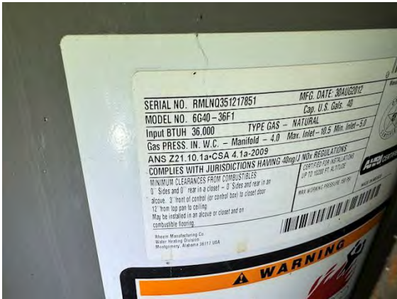
Unit # 10 Water Heater:
