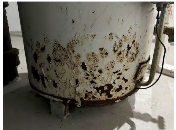
Unit # 12 Water Heater:
