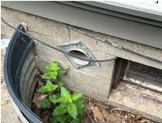
Laundry Facilities: MISSING VENT COVER
