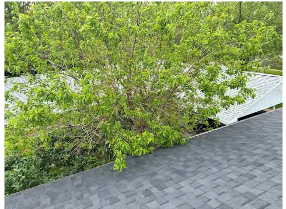
East Building Roofing: TREE BRANCHES IN CONTACT WITH ROOF
