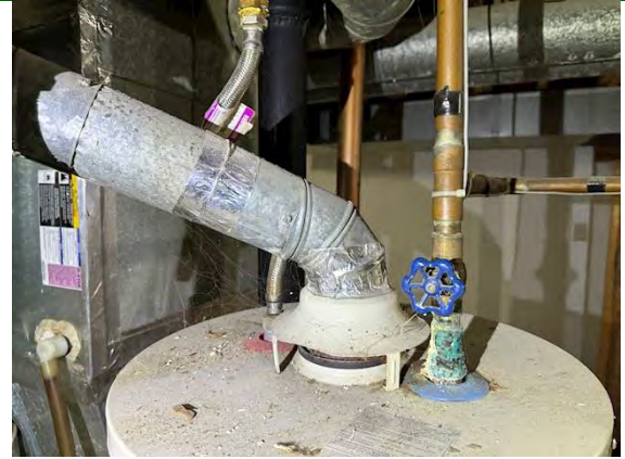
Unit # 8 Water Heater: NOT ENOUGH VERTICAL RISE
