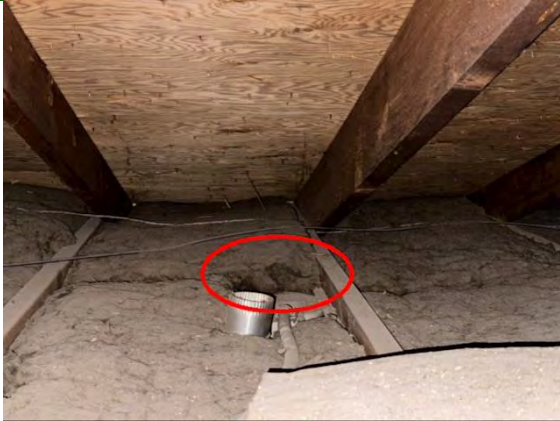
East Building Attic Insulation: MOISTURE STAINING IN INSULATION AROUND BATHROOM VENT
