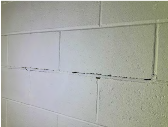
Unit # 4 Interior Foundation: GROUT CRACKS
