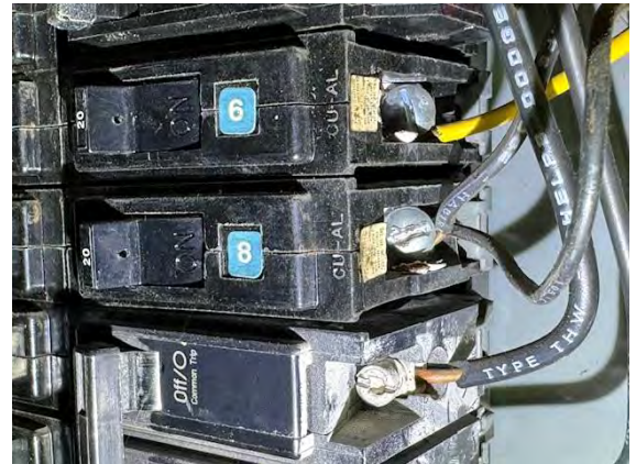
Unit #9 Electrical: DOUBLE TAPPED BREAKER
