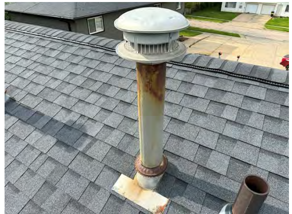
Unit # 7 Draft Control/Vent:
