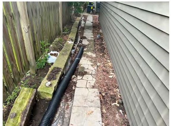
North Building Roof Drainage System: DAMAGED PIPING
