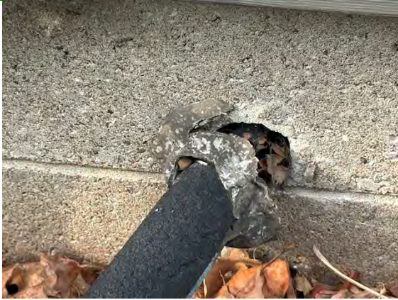
North Building Exterior Surface: UNCAULKED PENETRATIONS
