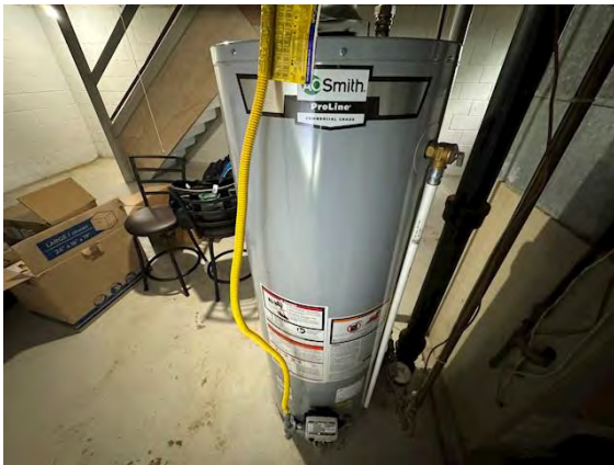
Unit # 3 Water Heater:
