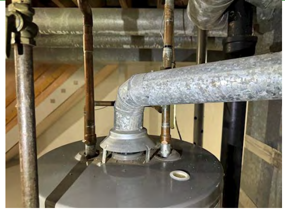
Unit # 11 Water Heater:
