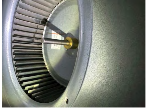
Unit # 11 HVAC Distribution:
