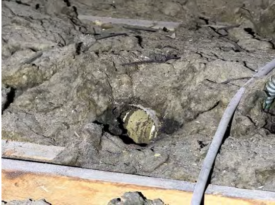
North Building Attic Insulation: MOISTURE STAINING INSULATION
