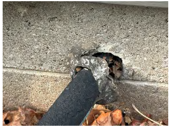
North Building Exterior Foundation: AC LINE PENETRATING FOUNDATION
