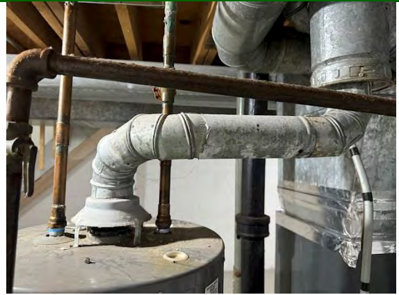
Unit # 13 Water Heater:
