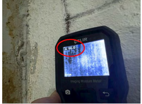
Unit # 1 Interior Foundation: MOISTURE LEVEL 96%
