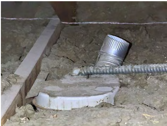
North Building Attic Ventilation: BATHROOM VENT TERMINATING IN ATTIC
