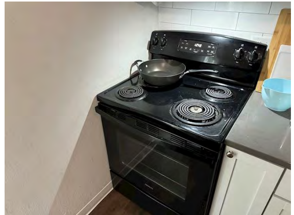
Unit # 3 Kitchen: OVEN INSTALLED IN DIRECT CONTACT WITH DRYWALL
