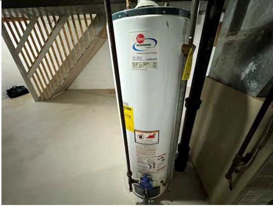
Unit # 15 Water Heater:
