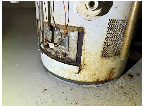
Unit # 9 Water Heater: COVER PLATE MISSING
