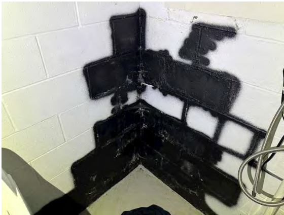
Unit # 3 Interior Foundation: PAST REPAIRS
