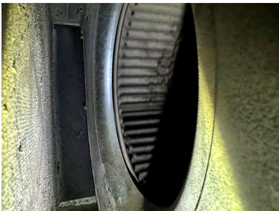
Unit # 15 HVAC Distribution: DIRTY BLOWER FINS
