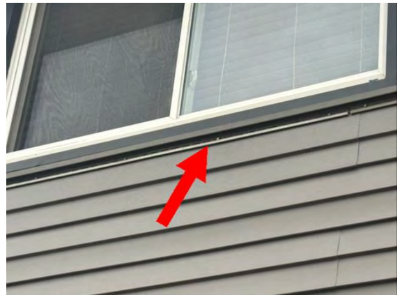
West Building Exterior Surface: MISSING TRIM WORK AROUND WINDOW
