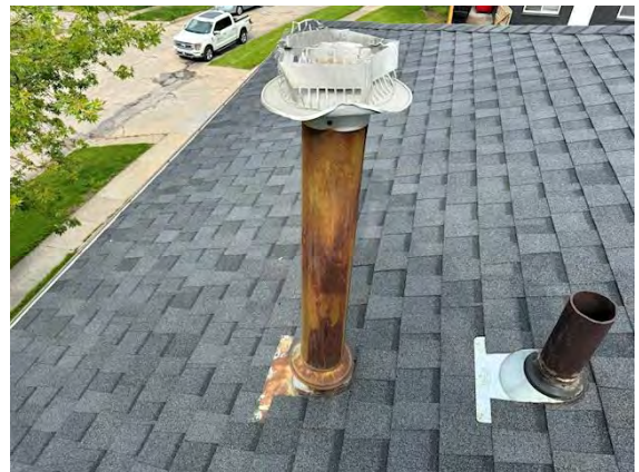
Unit # 15 Draft Control/Vent: MISSING RAIN CAP
