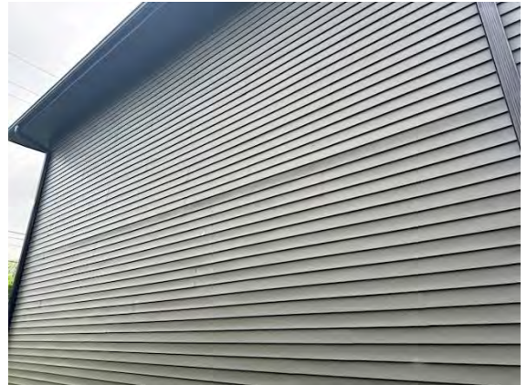
North Building Exterior Surface: BULGING IN SIDING
