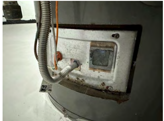
Unit # 13 Water Heater: MISSING COVER PLATE
