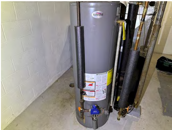
Unit # 4 Water Heater:
