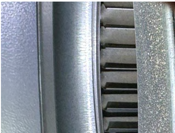
Unit # 7 HVAC Distribution:
