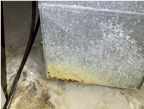
Unit # 5 HVAC Distribution: RUST BUILD UP
