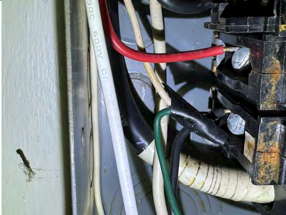
Unit #8 Electrical: SPLICING WITHIN THE PANEL
