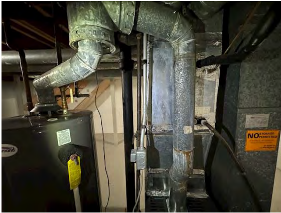
Unit # 11 Draft Control/Vent:
